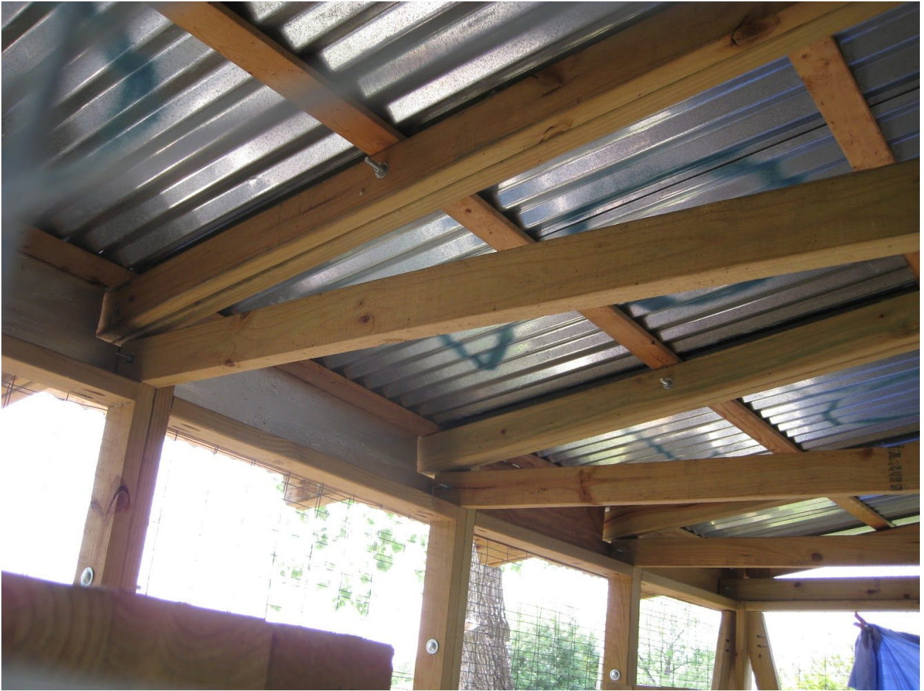
Interior shot showing truss, roof module, blocking wood, roofing and stringer details.
