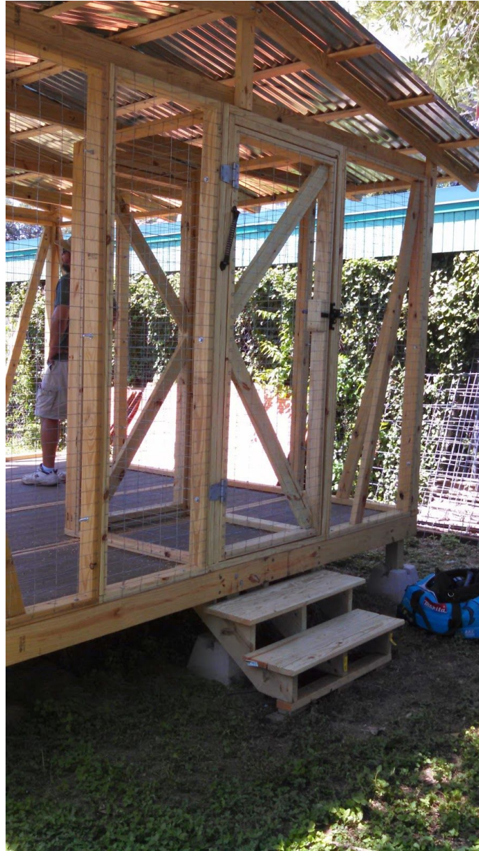
Photo showing modular sections, airlock and stairs.. Photo was taken before second layer of wire screening was added.
