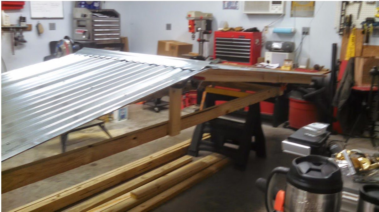
Photo showing an end pair of roof panels under construction. Note king post and truss bottom component.
